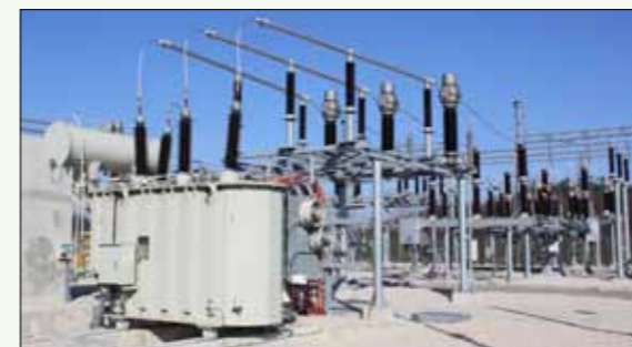
LG Chem Ltd. Yeosu Plant LDPE
